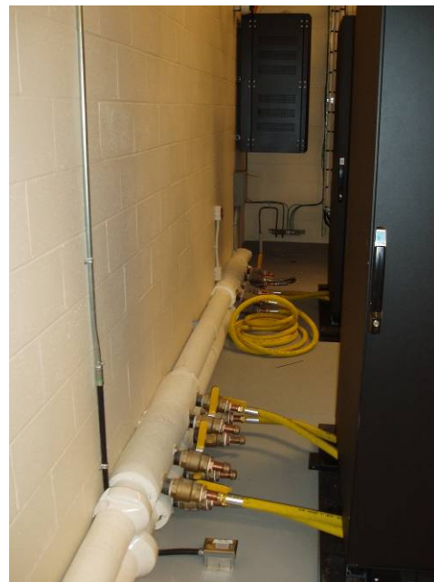
Manifold for Chilled Water
