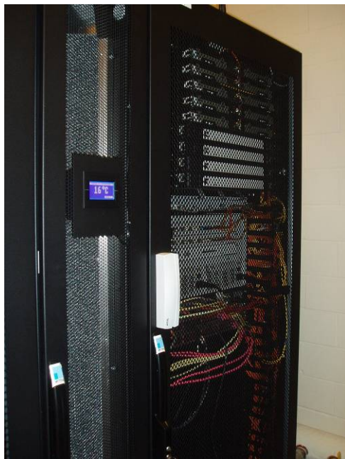
Cabinets and Cooling Panel
