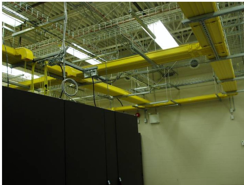
Cable Management System
