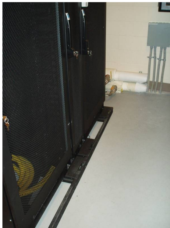
Equipment Racks on Seismic Isolation Pads
